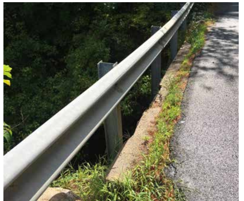
Road crumbling on Emery Mills Bridge. PHOTOS BY JOANNE BARGIONI
