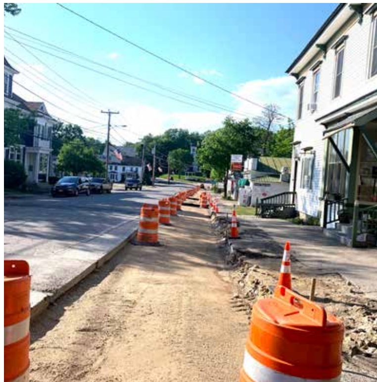
The sidewalks along Main Street in Limerick were recently dug up to replace the sewer lines as part of a rebuilding project.
