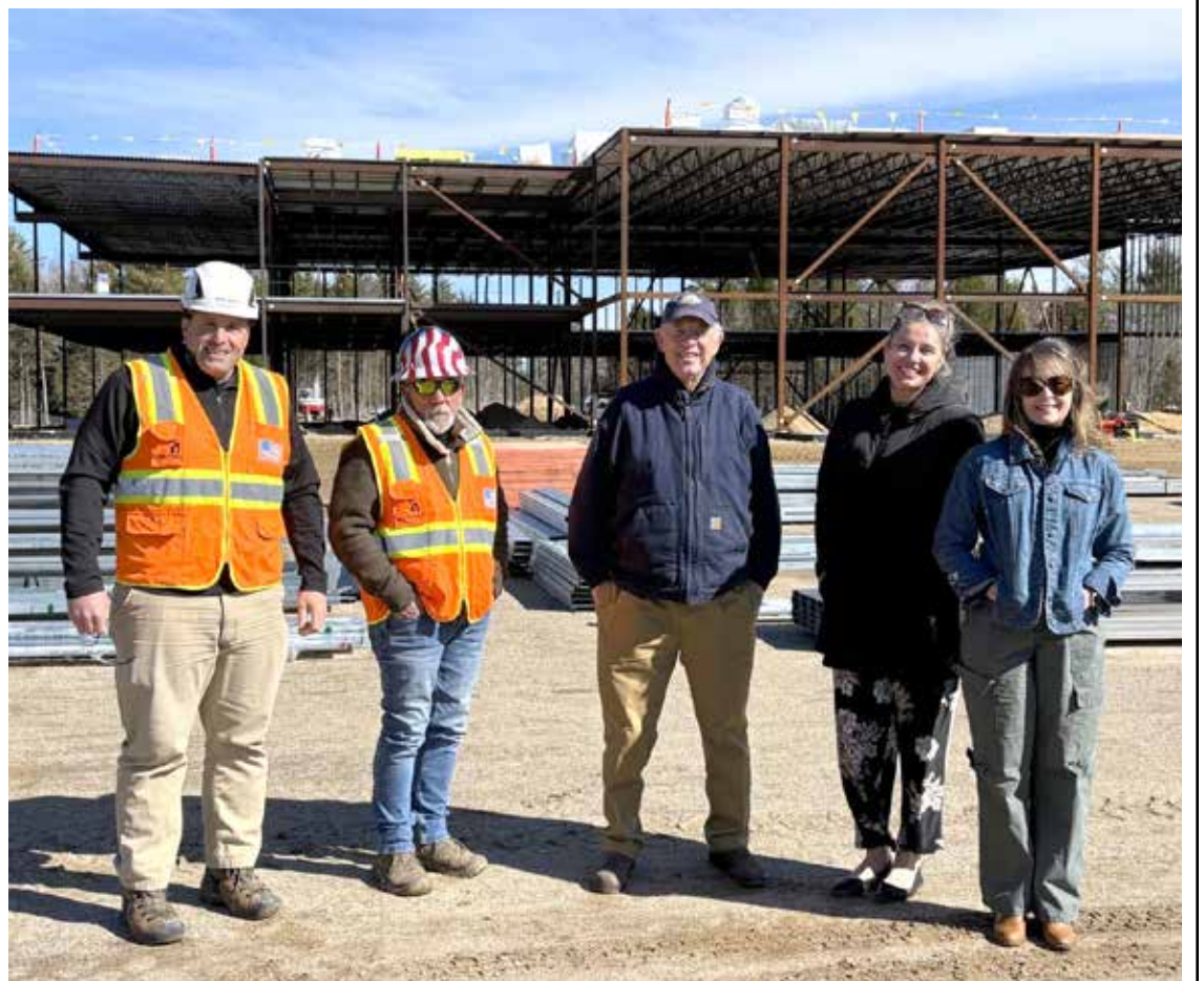
First County Foundation (FCF) board members recently had an up close look at York County government's two building projects – a first responder training center and a substance use recovery center – under construction on Layman Way in Alfred. FCF is the charitable arm of the county government, and looks to help fill in the gaps – from equipping a kitchen to supplying beds for the recovery center – through fundraising. The steel has been hung for the training center, and the footings for the recovery center are to soon be installed. Pausing for a photo following their tour were, from left, Senior Project Manager Tim Sommers and Superintendent Steve LaPointe of Landry French Construction; FCF Chair Billy Shore, who also serves on Kennebunkport Fire Department, along with FCF Board Member and Kennebunk Police Officer Candice Simeon and FCF Board Member and Sanford Housing Authority Executive Director Diane Small. PHOTO BY RACHEL STANSFIELD/YORK COUNTY GOVERNMENT
