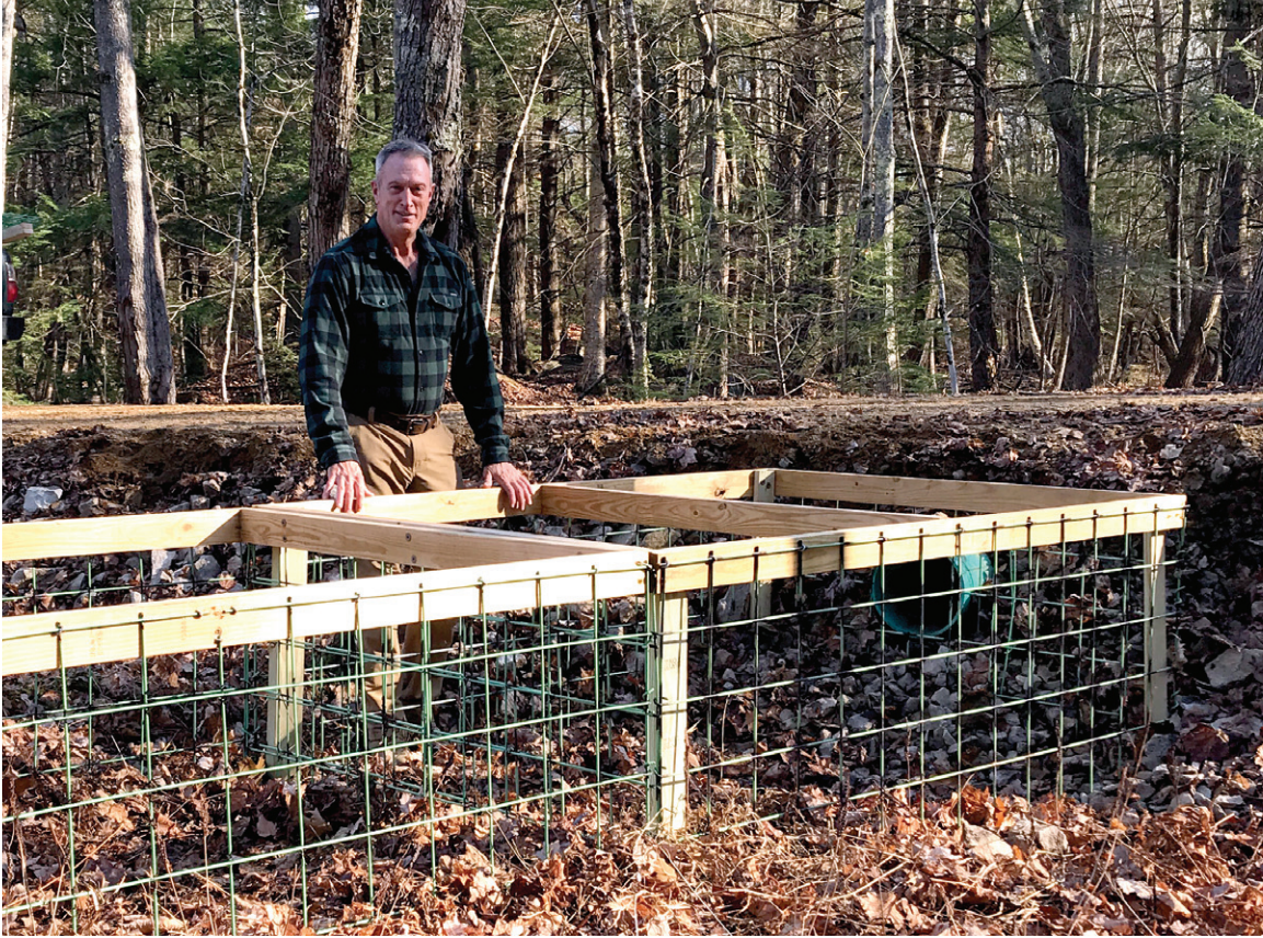
Skip Lisle with his latest 'Beaver Deceiver' installation along Sanford's improved Rail Trail, in background. PHOTO BY KEVIN MCKEON.
