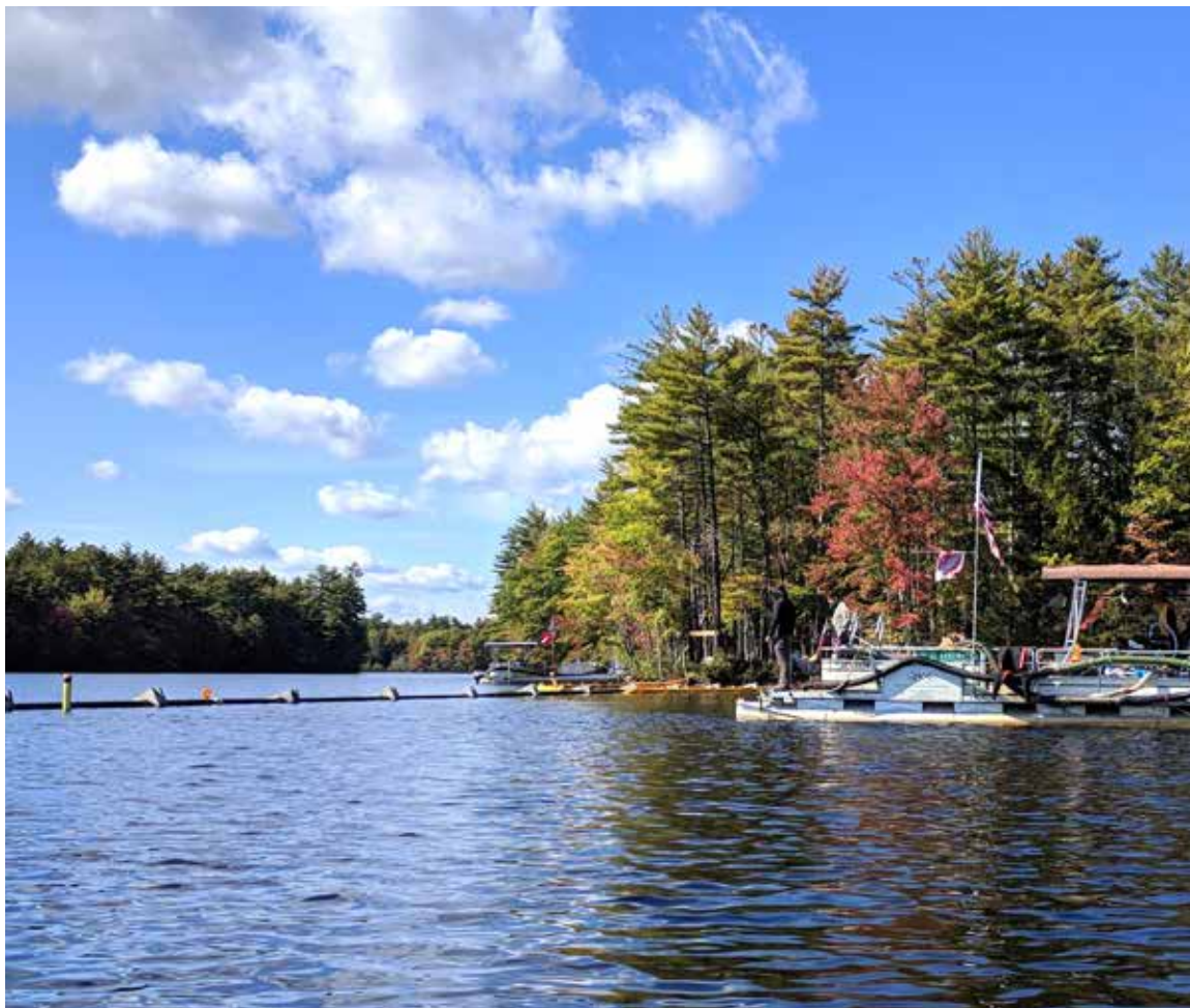
On Oct. 5, after the lowering of the level of Lake Arrowhead, the Lake Arrowhead Community Public Works crew began installing a water pipeline across the lake as part of a community water system upgrade. This photo shows the pipe with attached weights coming into the lake on the north side from Leasure Lane, in Limerick, heading across to Old Portland Road, in North Waterboro. The work is anticipated to take about a week to complete, at which time the lake level will be returned to the normal seasonal level.
