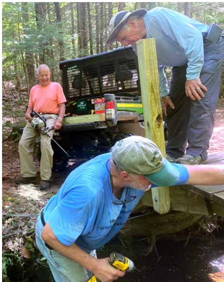
Hazen Carpenter, Kevin McKeon, and Thom Gagne repairing a woodland foot bridge along Mousam Way North Trail. PHOTO BY SAM PARADY
