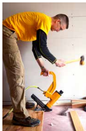
Jeff St. Laurent installing hardwood flooring during a recent Habitat for Humanity project.
