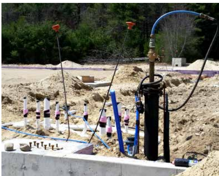
Work is underway on the foundation of a brand new Plummer's Ace Hardware and Family Dollar Stores at their former location on Route 202 in Waterboro. PHOTO BY BRIGIT MCCALLUM
