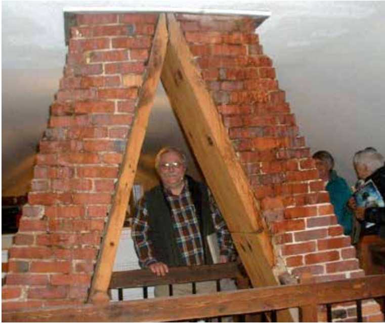
Alfred Historian Bruce Tucker examines the unusual brick structure in the attic chimney of an old York County Jail in Alfred. PHOTO BY ALLISON WILLIAMS
